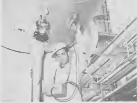
USING A Penetron with standard head, J. Cross, EIG senior engineering assistant, measures the shell wall thickness on a drum. Inspectors are trained to use a variety of standard and special tools.
